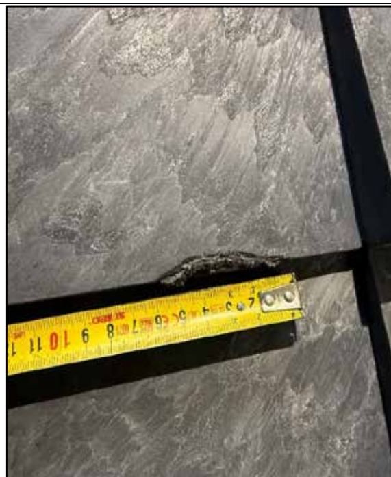
Figure 4: Damage investigation on the surface of the specimen
